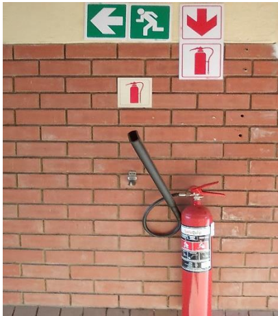
Valid fire extinguisher & SABS approved signage
