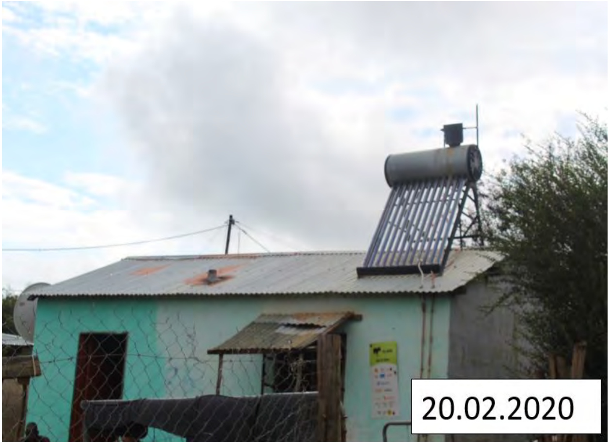
Solar guizers at Himeville Township
