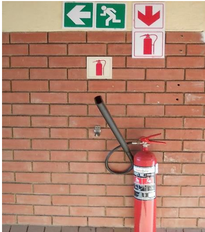
Valid fire extinguisher & SABS approved signage
