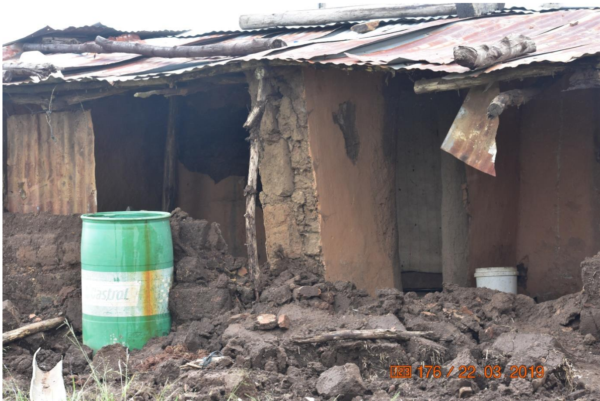
Figure 29- House that collapsed during February- March 2019 heavy rain
