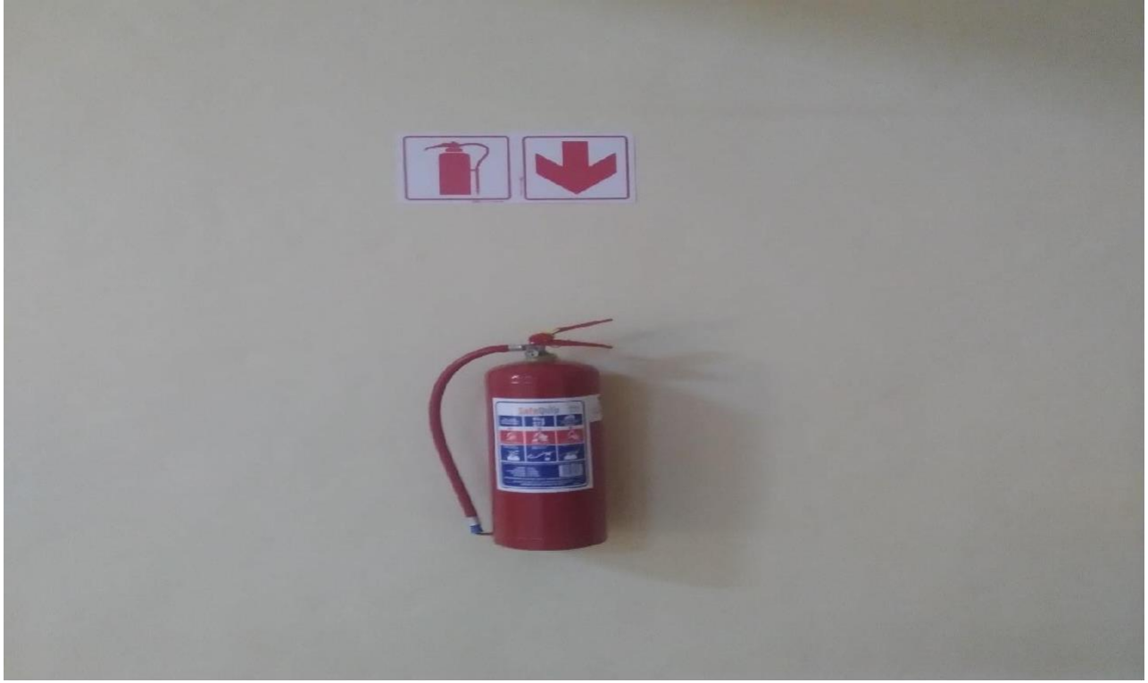
Fire Extinguisher and its Signage.
