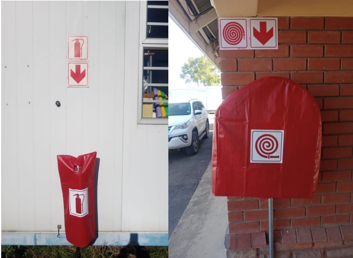
Fire extinguisher and Fire hose reel Covered with PVC covers
