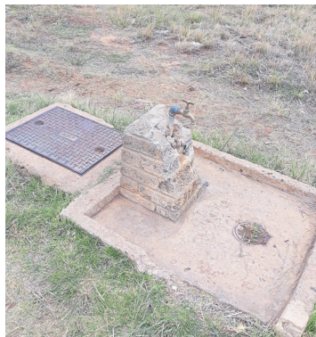
PHOTO: SUPPLIED A vandalised dry tap at Zwelitsha village.
