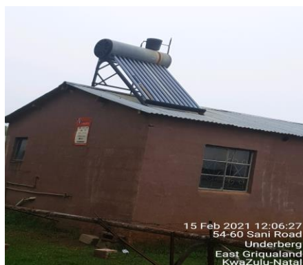
Solar guizers at Himeville Township
