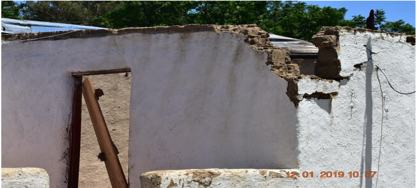
Roof blown away by wind
