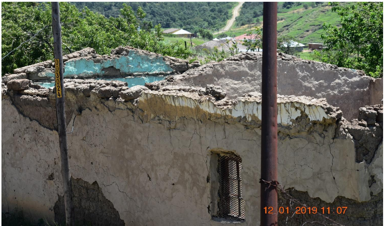
House its roof blown away
